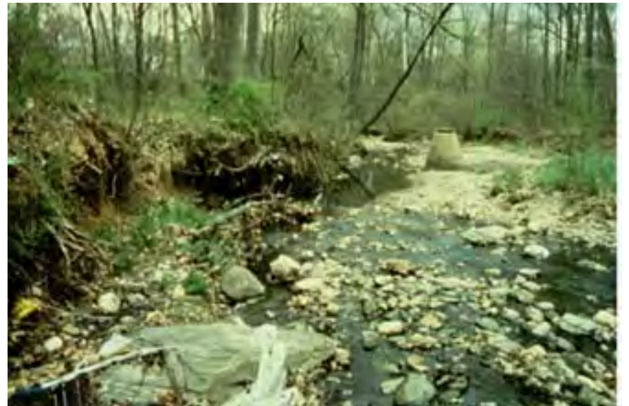
This stream has a 30% impervious cover. The size of the stream channel has increased by five to ten times.
