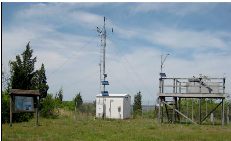
Figure 23. Meteorological station at Potter Cove showing the wooden platform and aluminum tower where the sensors are located for the collection of atmospheric data.
